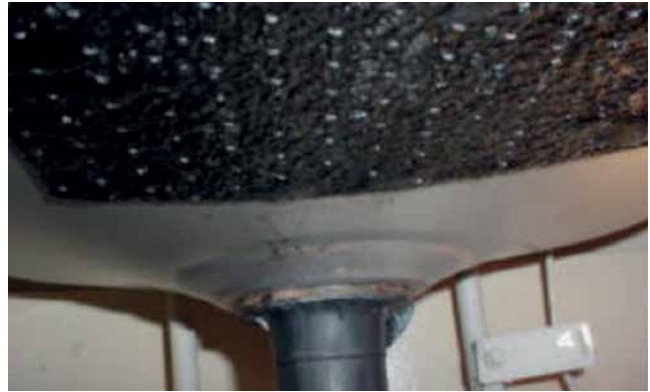
Asbestos containing sink pad.
