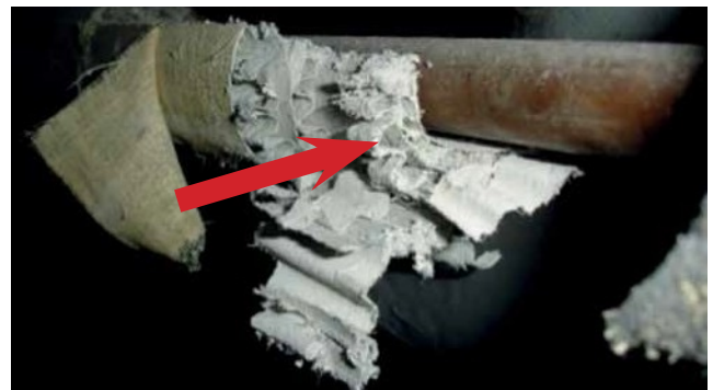
Asbestos corrugated paper as insulation.
